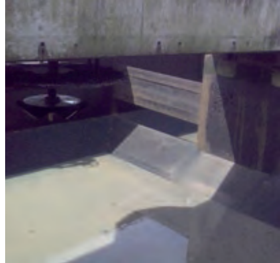
Activated sludge (AS) zone, empty to show surface paddle for aeration. Mike Dempsey
